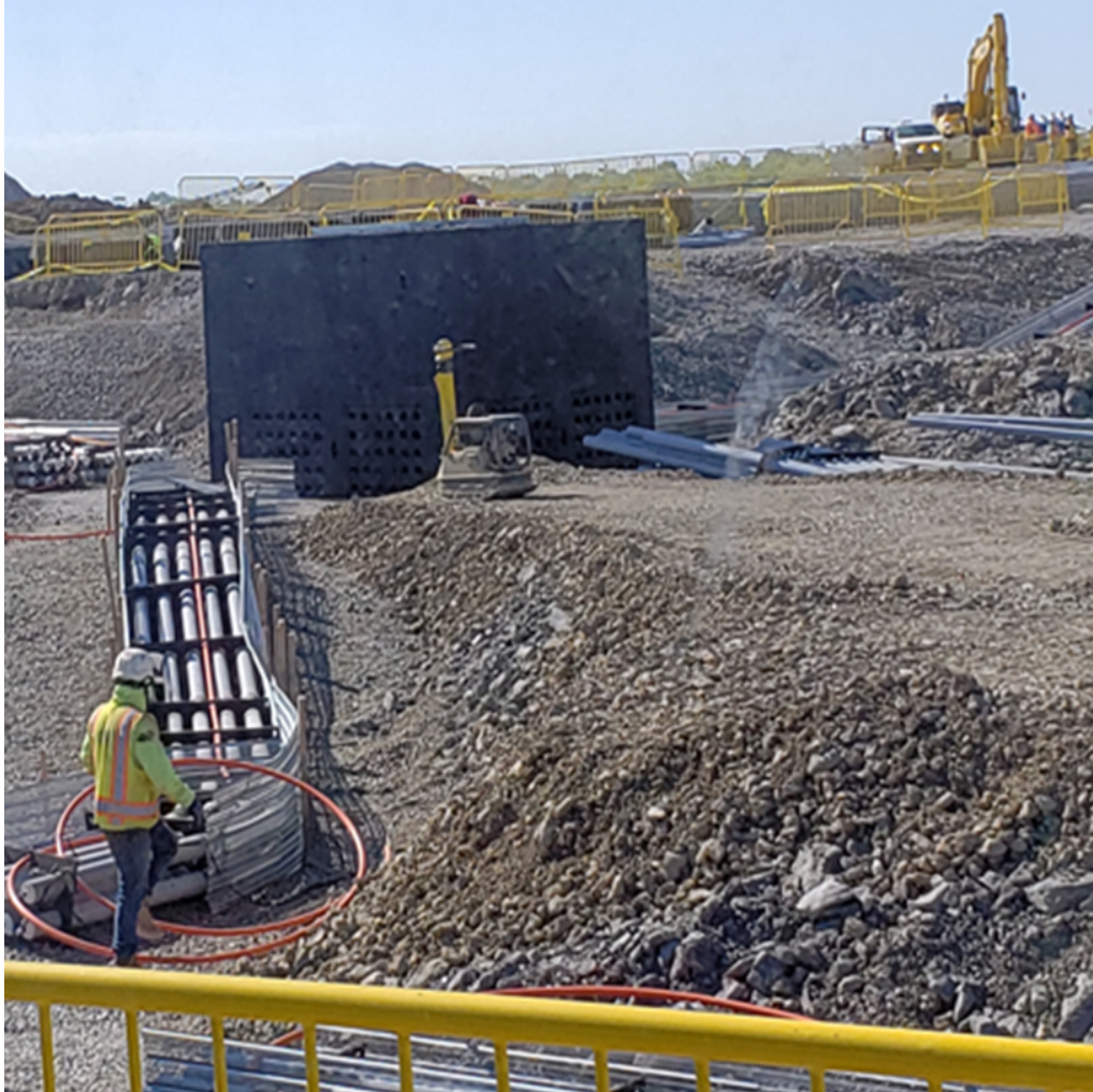
E-Infrastructure Solutions data center project
