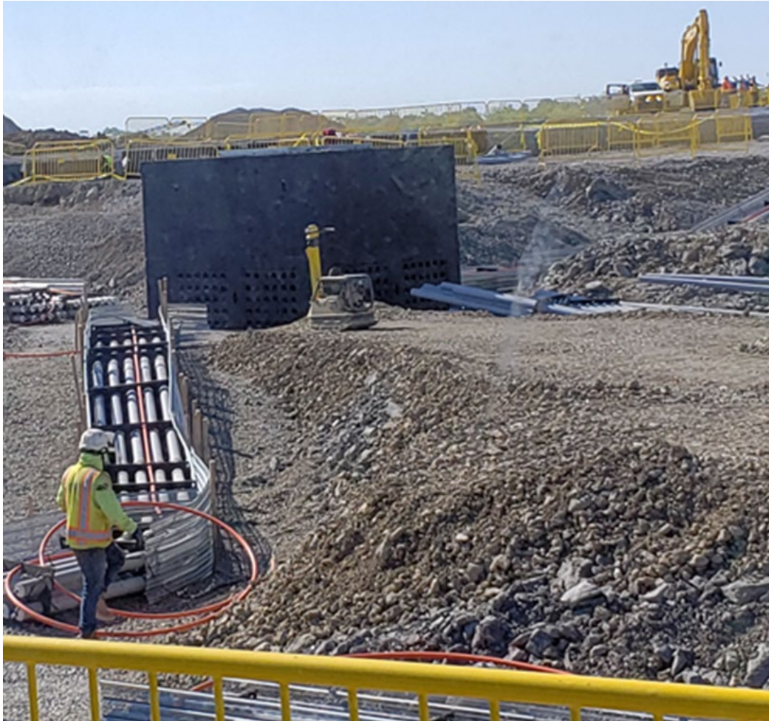
E-Infrastructure Solutions data center project
